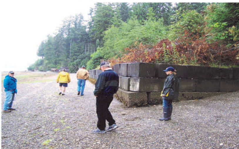
A prime example of an encroached bulkhead commonly found along Puget Sound beaches.
